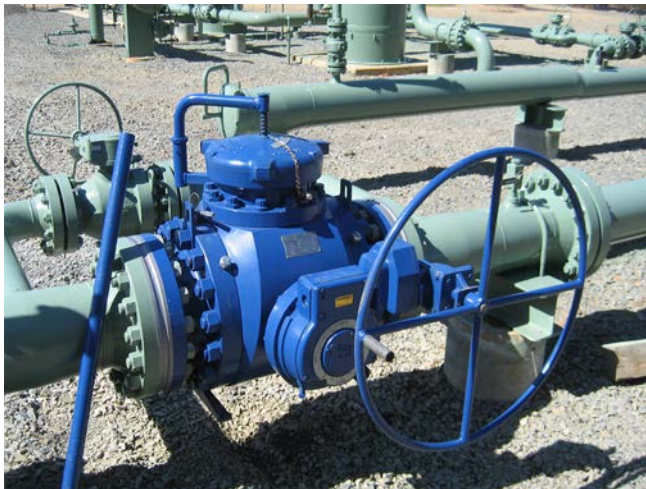
Figure 1. A 10 in. Argus pig valve receiver station in Haynesville Shale Gas, Louisiana (USA).
